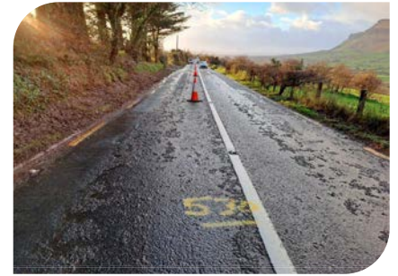
Existing N16 Pavement in Poor Condition
